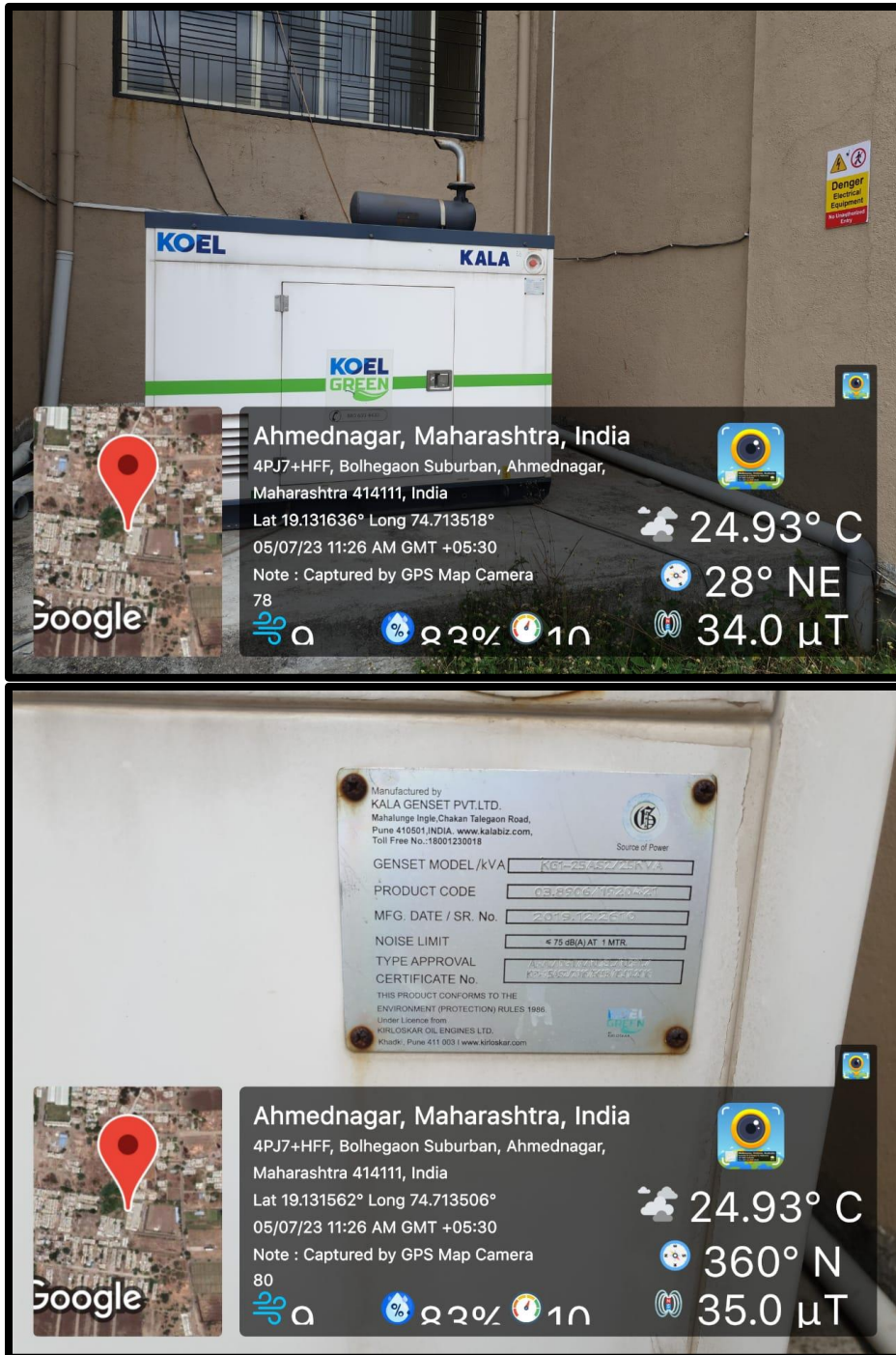
25KVA Generator Set for Power Backup
