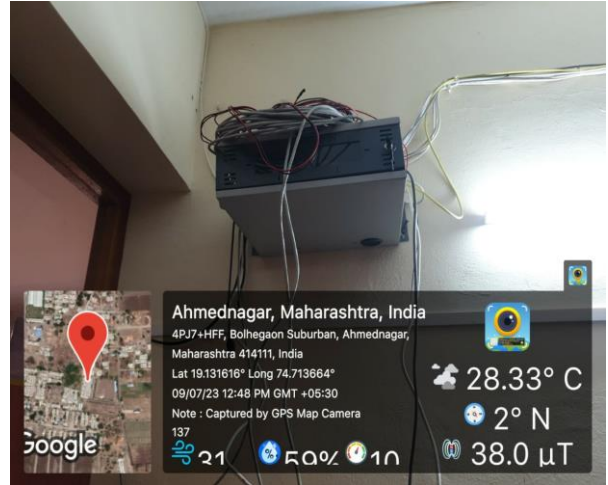
Internet Switch in Principal Cabin
