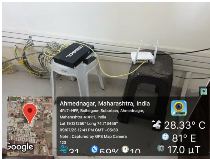
Internet Switch and WIFI Router in Computer Lab
