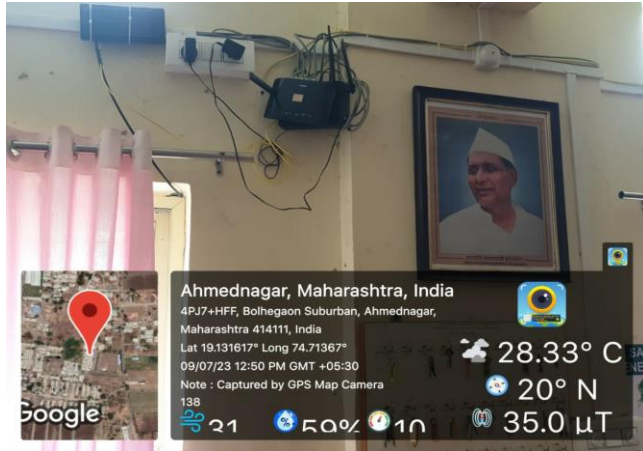
WIFI Router in Administrative Office
