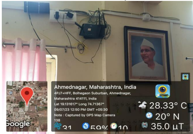
WiFi Router in Administrative Office
