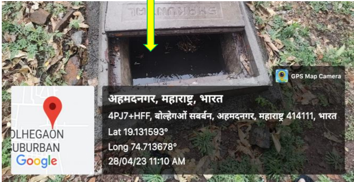
Rain Water Harvesting line chamber
