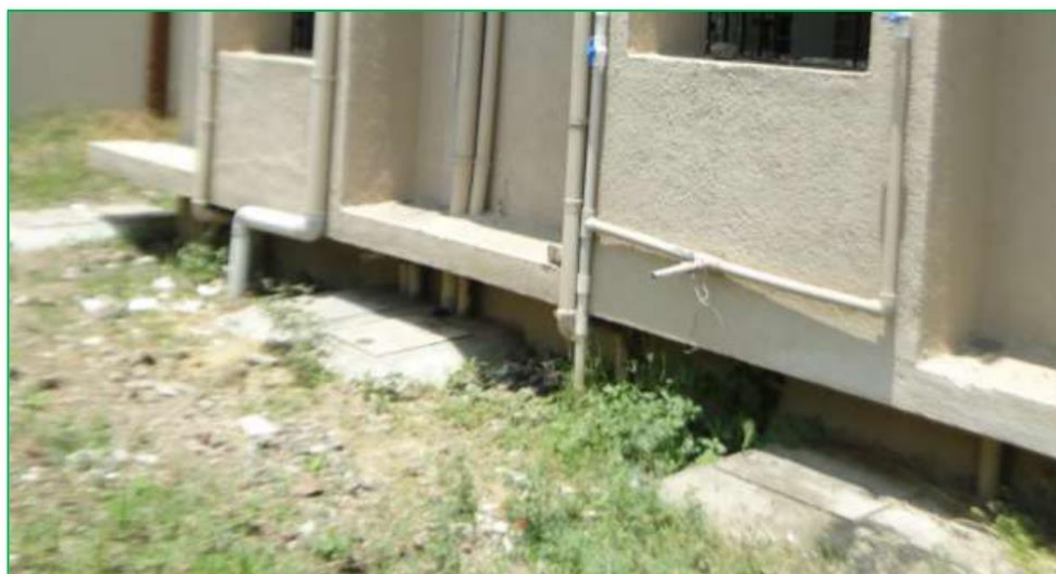
Liquid Waste Soak Pit
