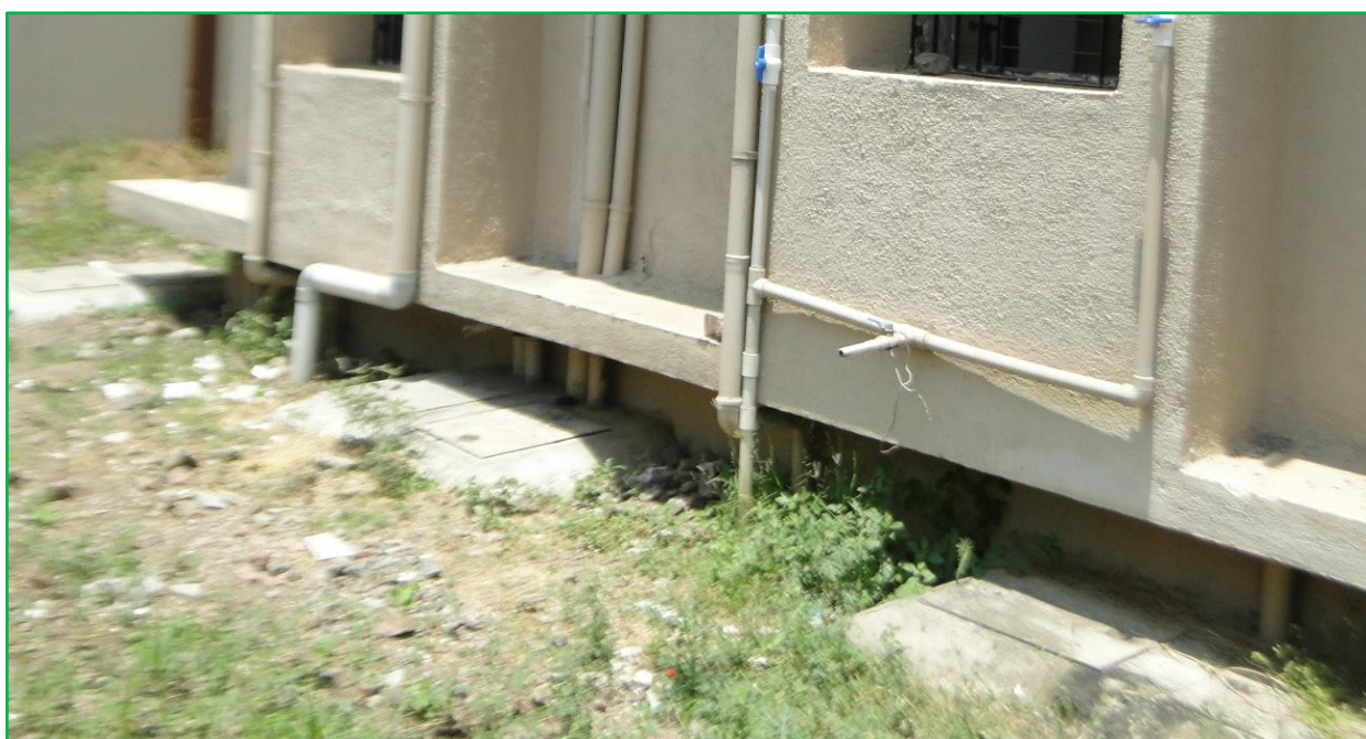
Liquid Waste Soak Pit
