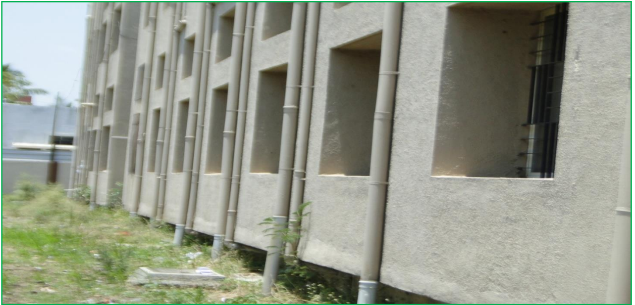
Rainwater Deposited Pipe
