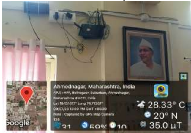
WiFi Router in Administrative Office
