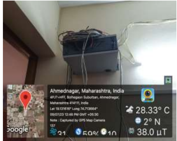
Internet Switch in Principal Cabin
