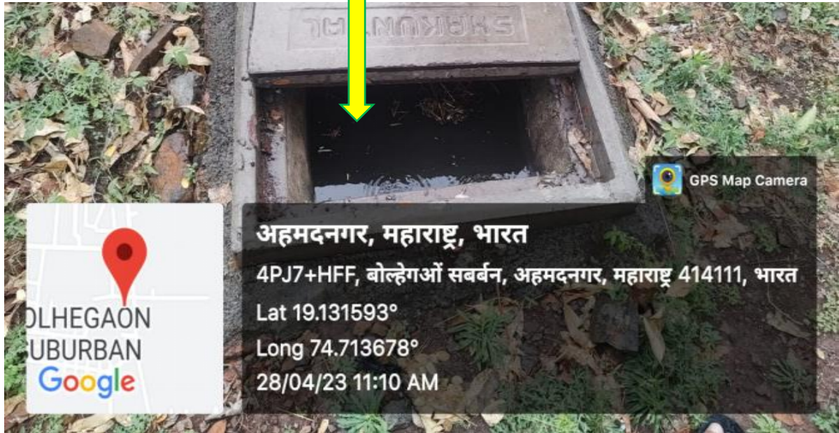
Rain Water Harvesting line chamber
