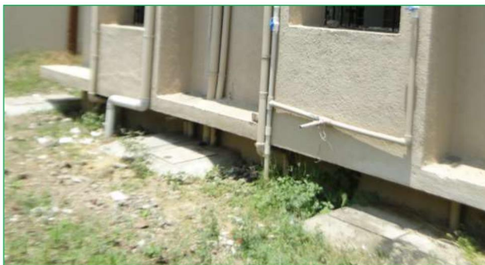
Liquid Waste Soak Pit
